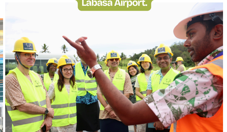
Fiji Airports Director Projects, Niranjwan Chettiar, provides an update to the delegation on runway strengthening works at Labasa Airport.
